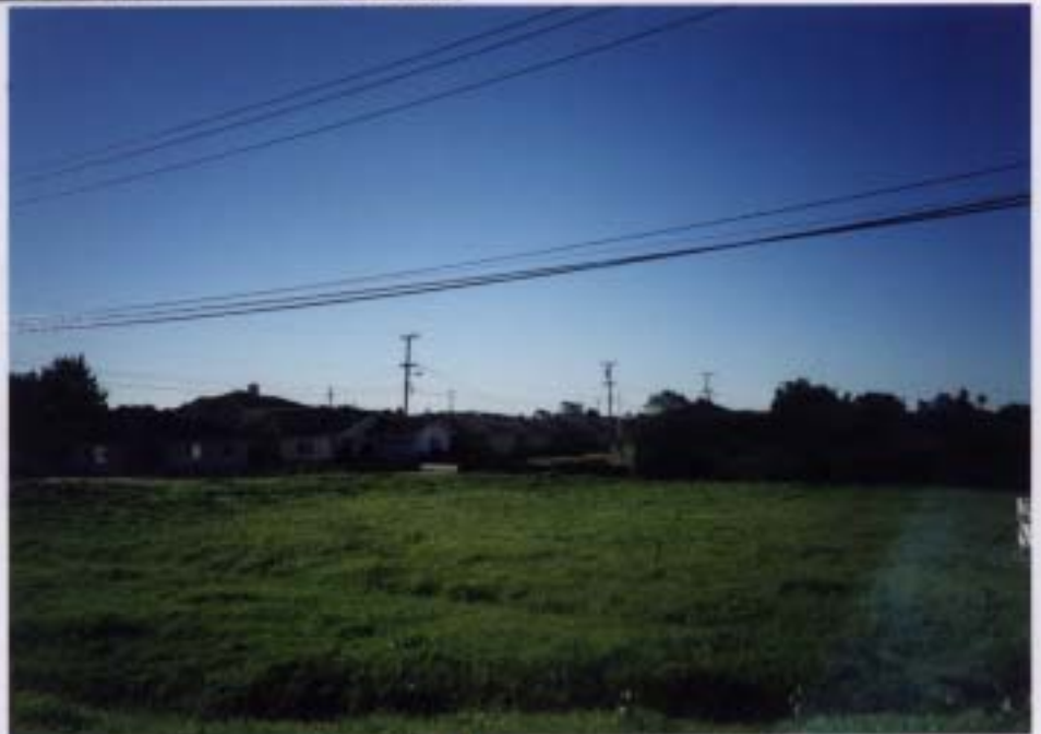
ELECTRIC POWER SERVICE ON WEST SIDE OF HIGHWAY 1 NEAR TEST WELL 4 AND GRAND PLACE
