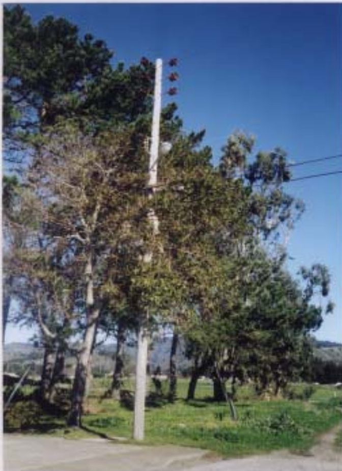
ELECTRIC SERVICE POLE NO. 7722 AT NORTHWEST CORNER OF CHESTERFIELD STREET AND ST. JAMES AVENUE 150' WEST OF TEST WELL 3
