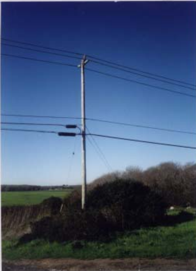
ELECTRIC POWER POLE NEAR TEST WELL 4
