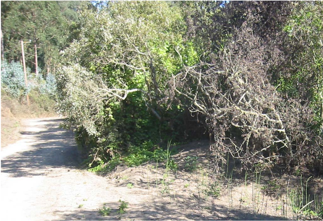
Road erosion adjacent to Denniston Creek
