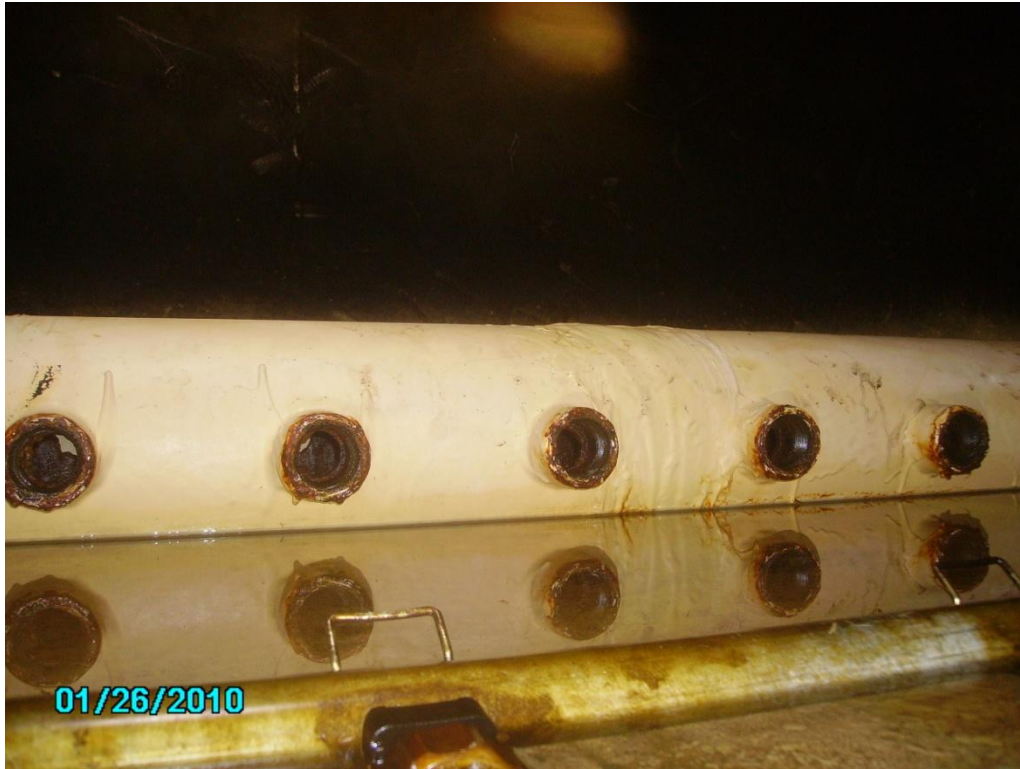
Photo 5. Rusted Lateral Connections in Filter 3
