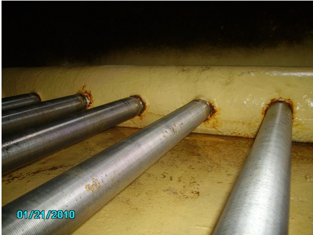
Photo 2. Corrosion of Steel Manifold at Connection Points of Wedgewire Laterals
